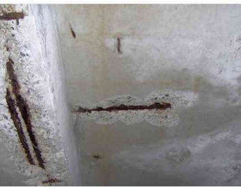
Corroding reinforcing steel and delaminated concrete.
