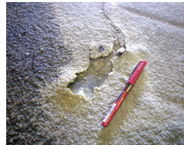
Delamination of suspended concrete slab membrane.
