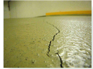
Cracks in a suspended concrete slab membrane.
