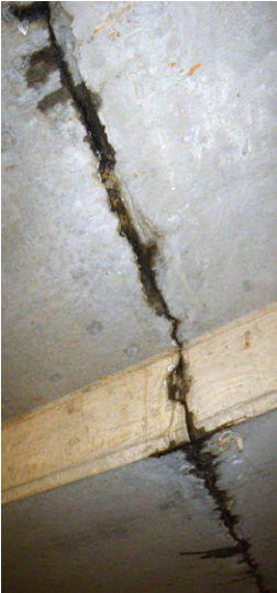
Water ingress through a crack in the concrete slab.
