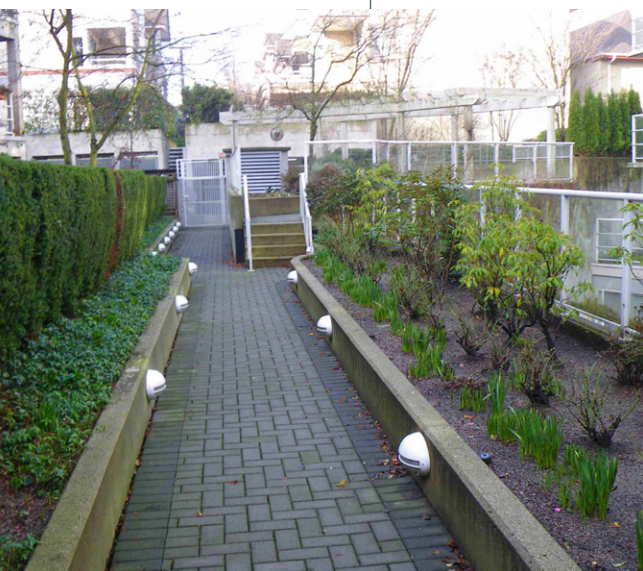
A typical courtyard at-grade assembly. This courtyard features many different types of overburden, making access to the underlying membrane difficult.
