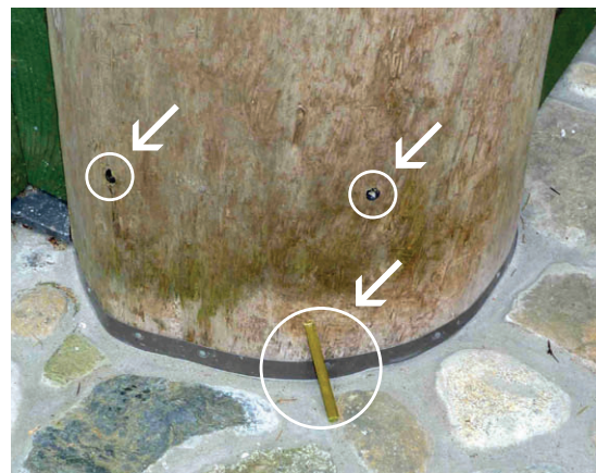
Installation of boron rods at base of post will provide greater resistance to decay. Boron rod shown leaning against base of post and locations where installed are highlighted by white arrows.
