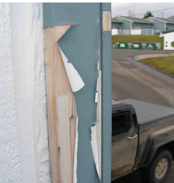
Paint peeling from wood substrate.
