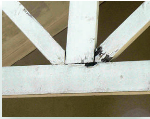
Open joints collect water and lead to deteriorated beams and columns at the connection.
