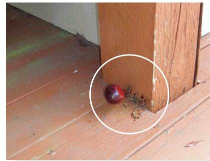
Probe reveals deteriorated wood post masked by solid stain.
