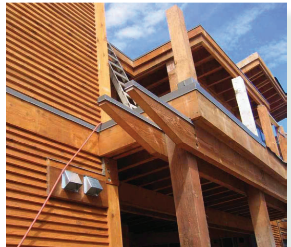
Metal cap flashing on exposed beam ends prevents water from collecting on the upper horizontal surfaces.
