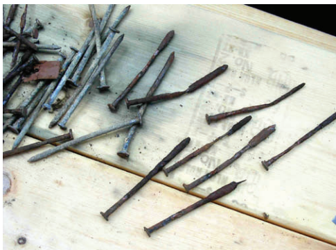
Corroded nails removed from deck boards.
