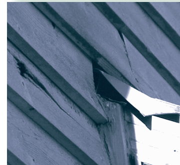
This wood siding has suffered irreparable, permanent damage that cannot be corrected by further paint or stain application. This could have been prevented through proper maintenance.
