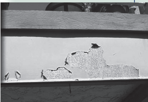
Paint peeling from a metal flashing: Good quality factory-finished metals would have better endurance than this site-painted metal flashing.
