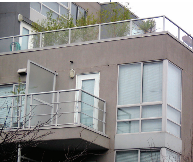
Windows and exterior doors deteriorate over time due to age, wear and tear and the weather, and require ongoing inspection and maintenance.
